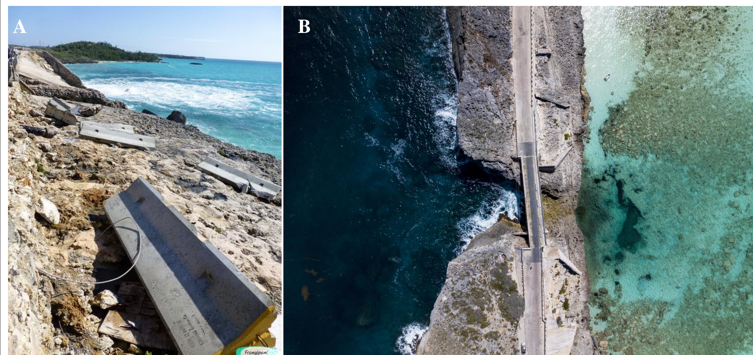
Figure 2 : A) depicts the damage caused by the Perfect Storm of 1991, wherein the roads were toppled into the Great Bahama. B) depicts the aerial image of the 12 feet westward displaced bridge
