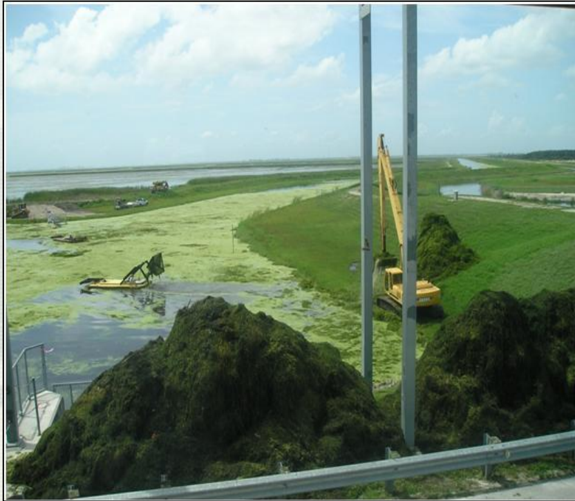
Accumulated debris at S-362
