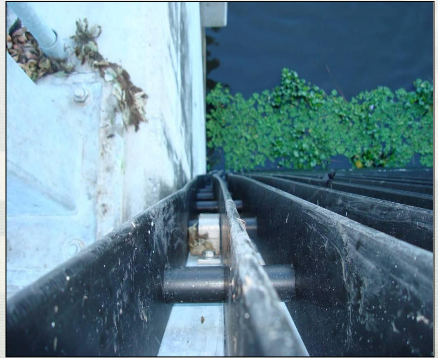
Deformed Trash Rack at S-319
