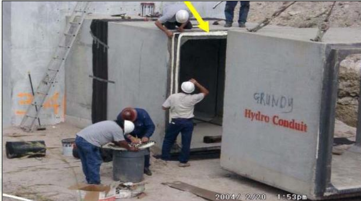
Segmented box culvert 8' x 8'
