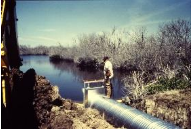
Figure 1. Culvert installation to restore a hydrologic connection to impounded mangroves, Indian River Lagoon, Florida, USA.
