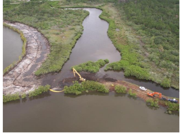
Figure 2. Excavation underway to remove an external dike and restore a hydrologic connection to impounded mangroves, Merritt Island National Wildlife Refuge, Merritt Island, Florida, USA, 2007.
