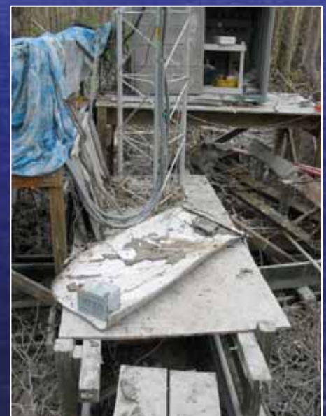
CO 2 tower in SRS-6 (100 m inland) after Wilma (see deposition).
