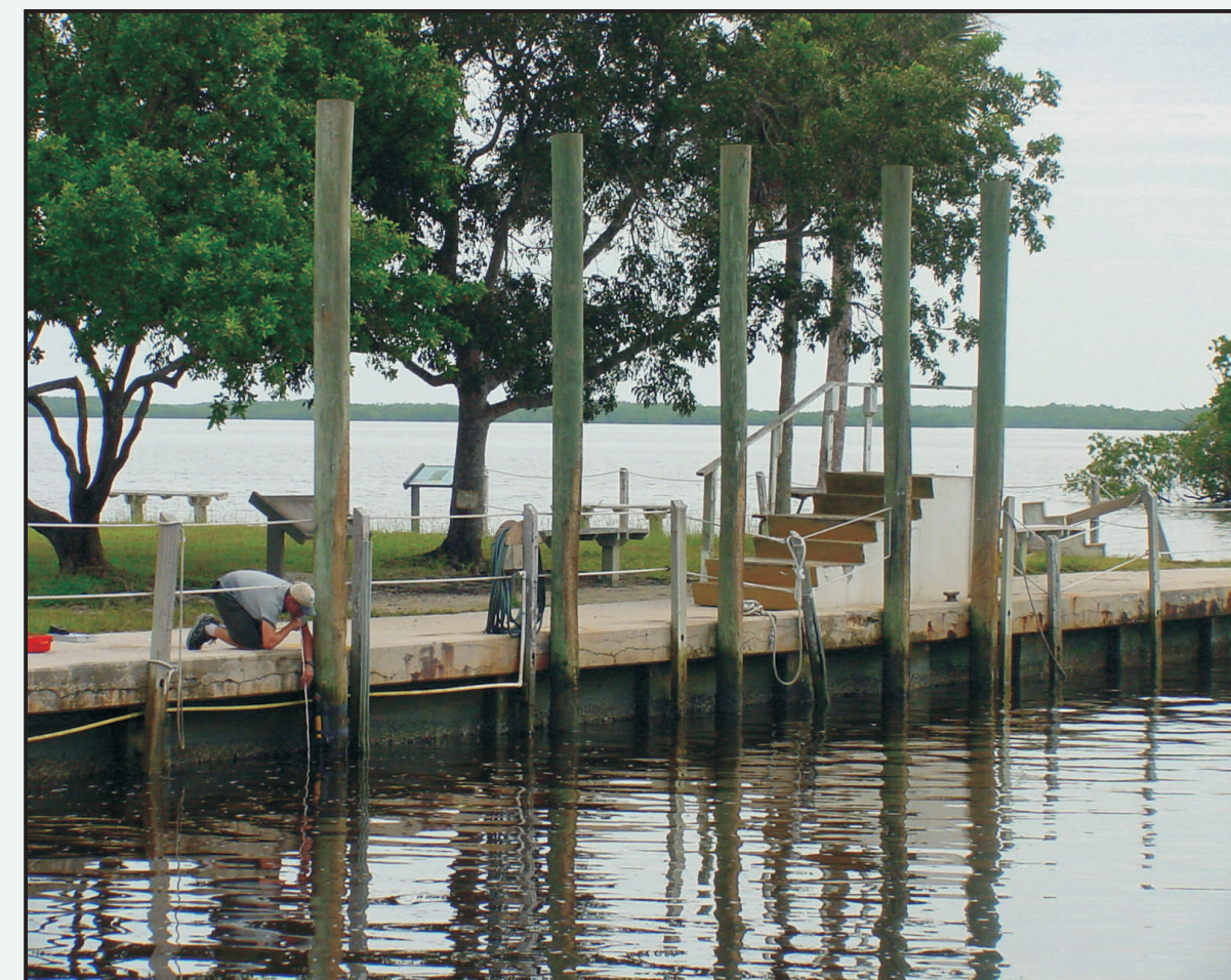
Figure 5. Water-level sensor deployment at WS_30 Everglades City.
