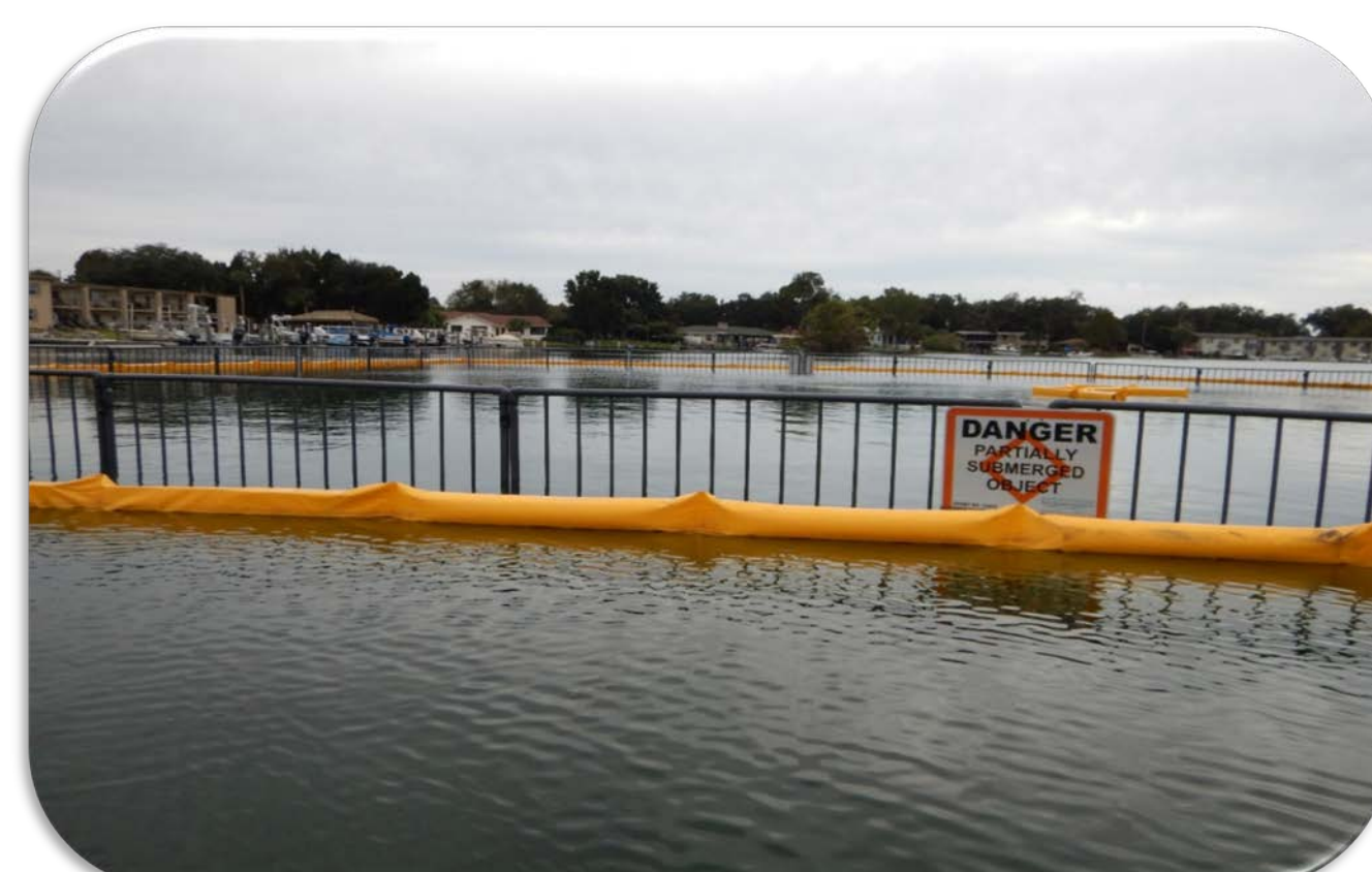
The PVC exclusion barriers were designed to conform to the bottom topography and extend >2' above mean high water to prevent manatees from accessing the restoration plots.
