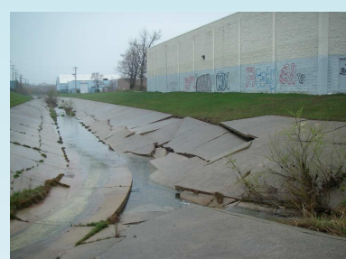
Figure 4. Damaged concrete lining in Holmes Avenue Creek.
