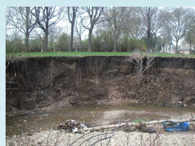
Figure 5. Bank erosion in the unlined portion of the KKR.
