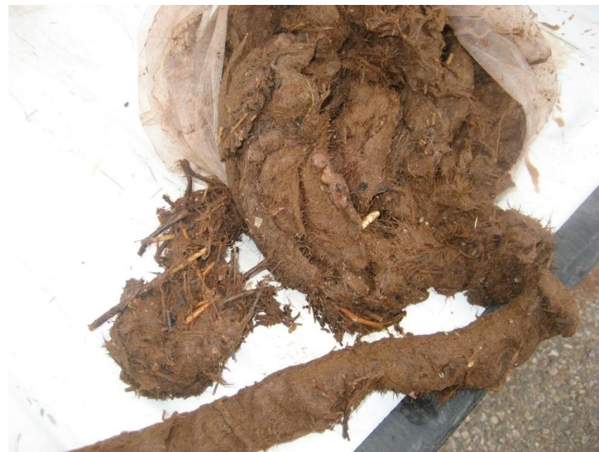
Salt cedar roots in adits at Abiquiu Dam
