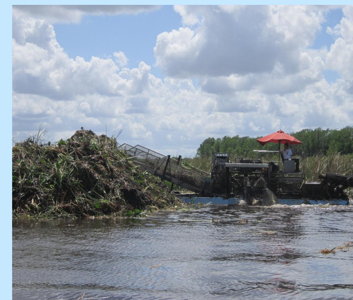
The removal of aquatic plants may be disposed of by creating large islands where the organic material may decompose over time
