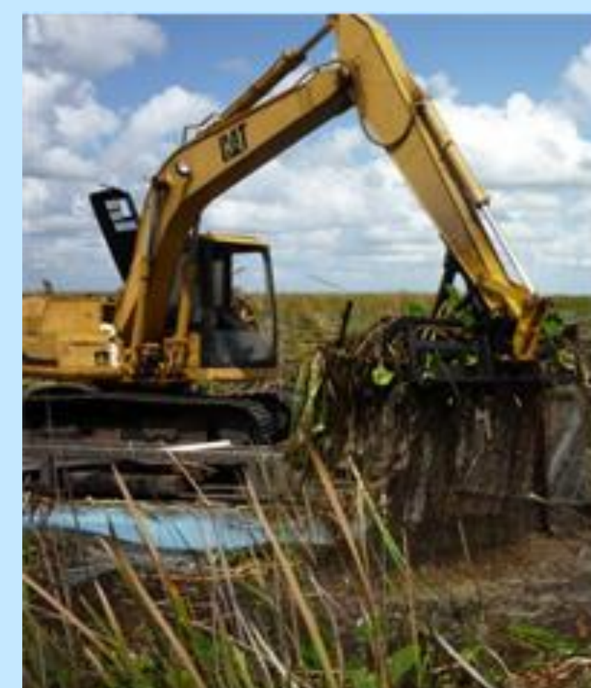
Barge-Mounted Excavators with a rake attachment are used to remove the bulk of the aquatic plant material
