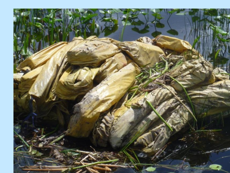
Silt curtains are out on site and ready to be deployed if turbidity levels get too high
