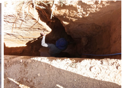
Very deep (2m) pipe infiltration
